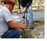
Solenoid valve installation
