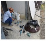
Drip laterals and drip tape
