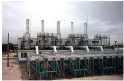
Sample diesel power generator
