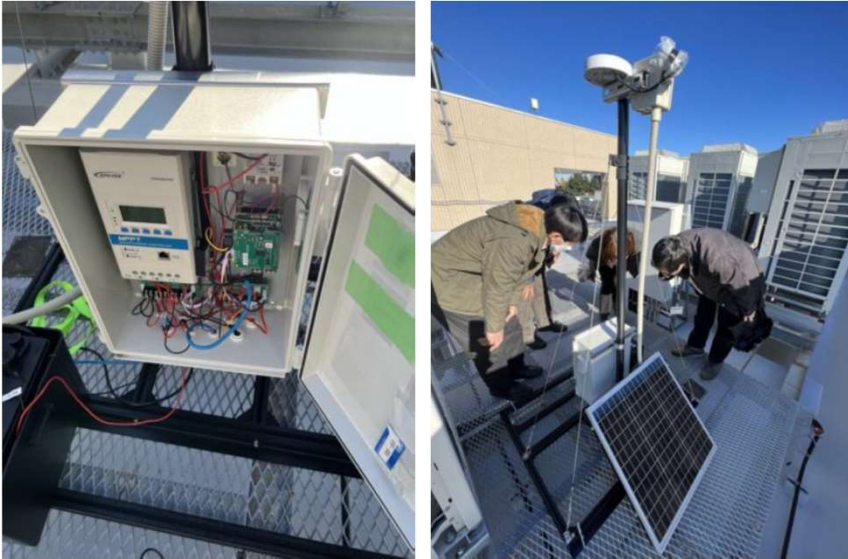
Visual IoT system installed at NICT
