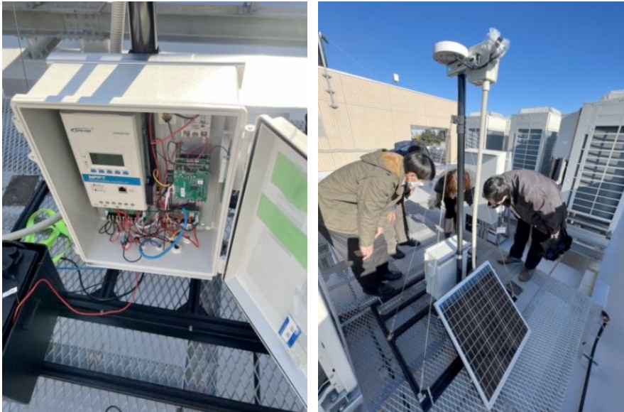
Viaul IoT system installed at NICT
